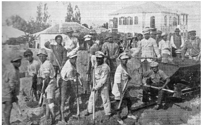
Page 644: 'The Baranovich Group' working on the construction of the Great Synagogue of Tel-Aviv, 1922.
